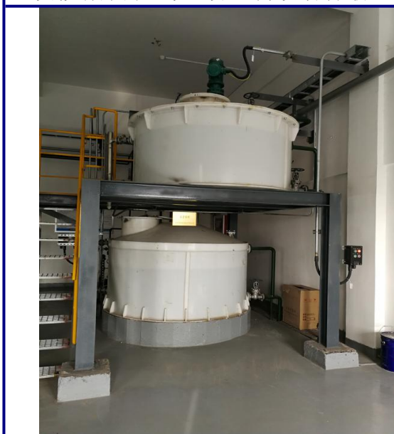
SNCR脱硝尿素溶液罐
